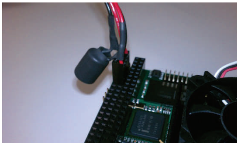
Figure 13) Example of a Capacitor installed across the main power input lines
